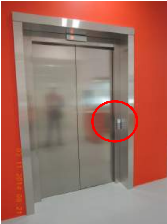
Figure 8 image of non-compliant lift call button installation
